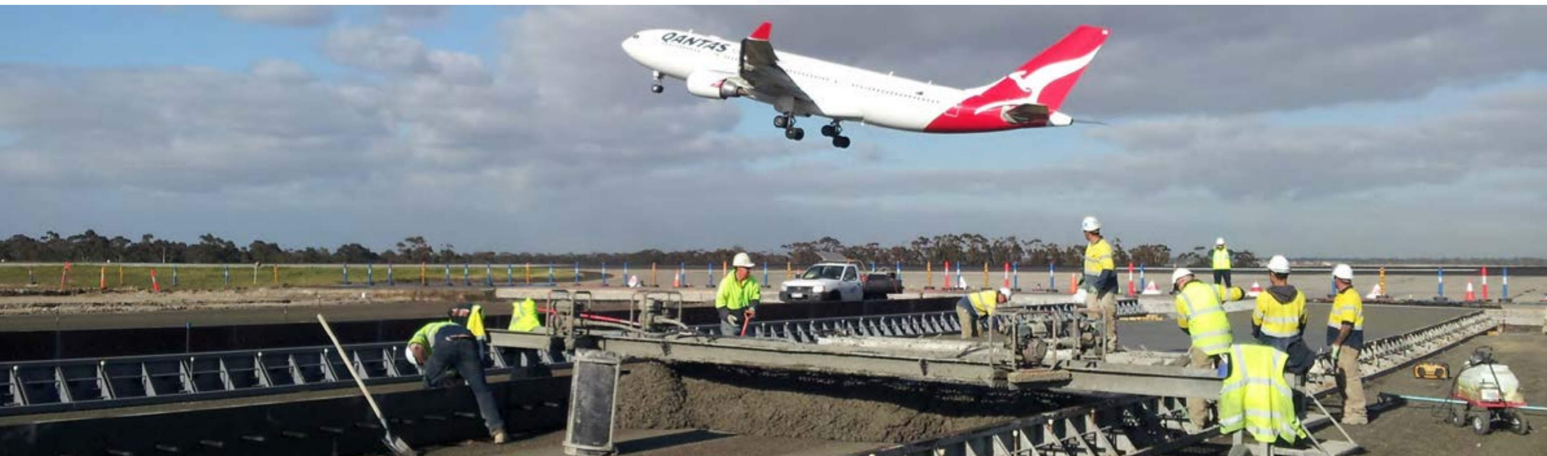
APAC staff and contractors lay concrete as part of the Victor Taxiway South construction works.
